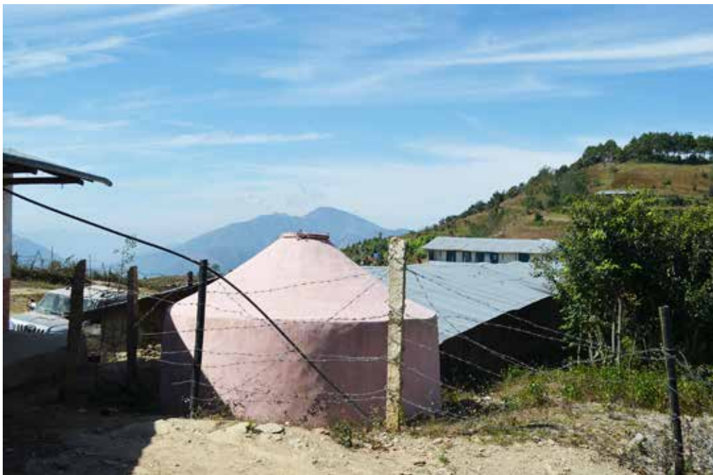
FIGURE 10. Rainwater harvesting tank in Ketuke.
