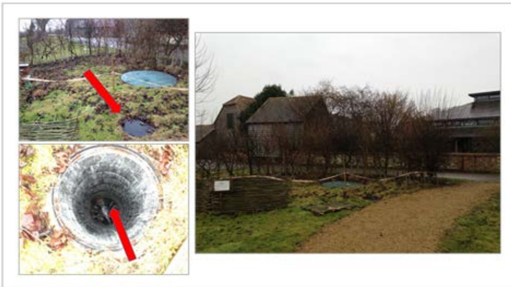
Plate 5 Location and sampling point for Tank 5, showing inspection cover and effluent sampling point within the inspection chamber
