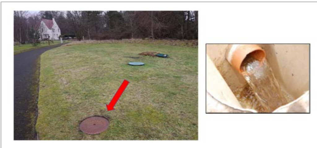
Plate 1 Location and sampling point for Tank 1, showing inspection cover and effluent sampling point within the inspection chamber
