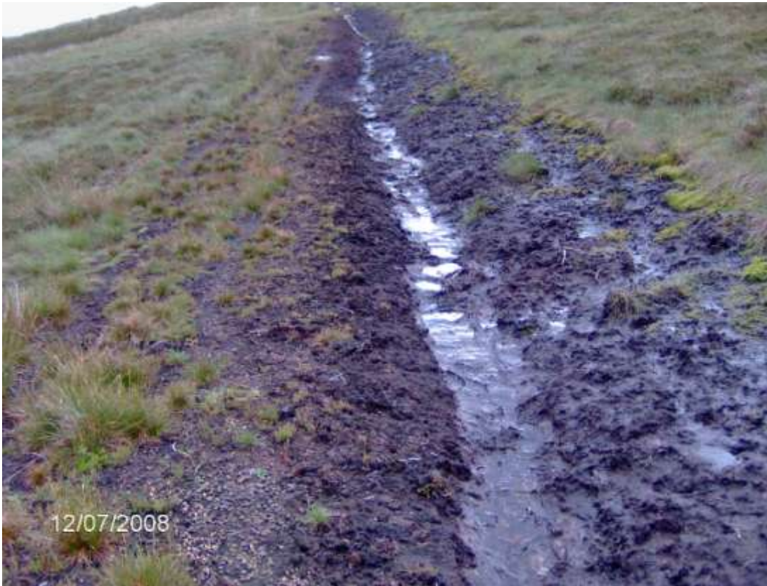
Plate C An example of track damage submitted to the Uplands Evidence Review. Photo: A. Peart, 2008.
