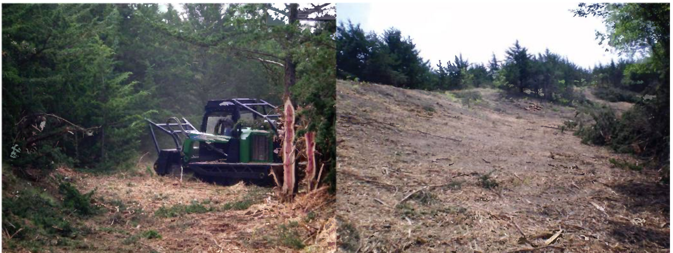
FIGURE 2 Forestry mulcher clearing the western side of the property. Cedars were cleared using a Gyro Trac model GT13 forestry mulcher in July 2008 (left). Post-clearing photograph shows bare soil and mulching residue (right). (Photographs courtesy of Matt Dollison.)
